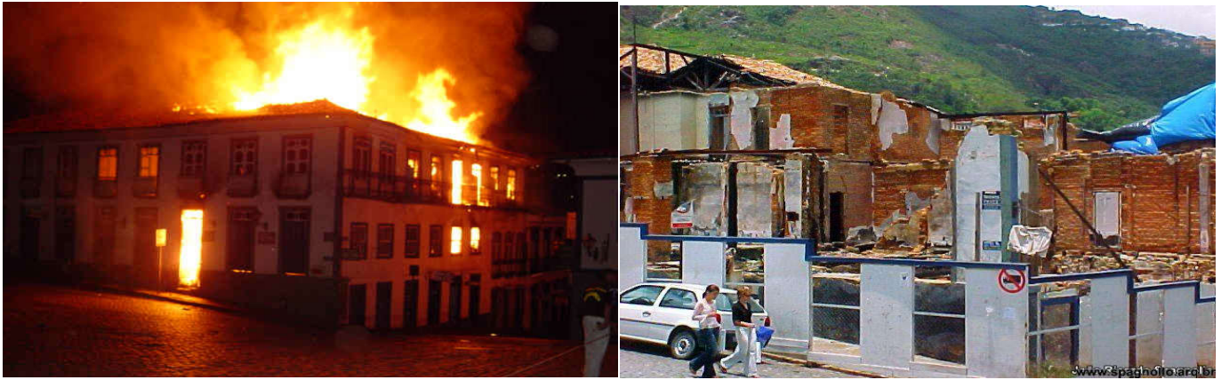
Figure 1. Images of the ancient Hotel Pilão, city of Ouro Preto, Minas Gerais State, Brazil (Oliveira, 2003)
