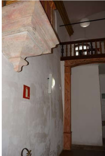
Figure 2. Deformation in the masonry resulted from the displacement of the armed rafter shear in the São José church in the city of Ouro Preto – Brazil
