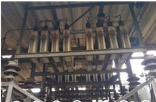
Fig1.Capacitor banks of the plant's substation [Author]
